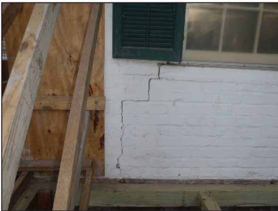
Figure 7. Severely cracked exterior wall on the Kellum-Noble House.
